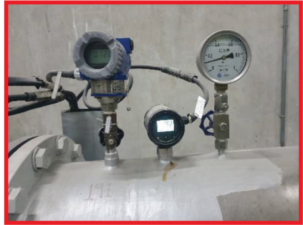
Level, Flow, Pressure, Temperature
