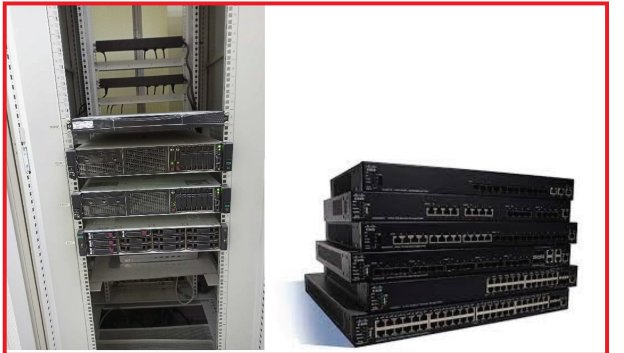
Our power system automation solutions are completed by our provision of SCADA servers and switches
