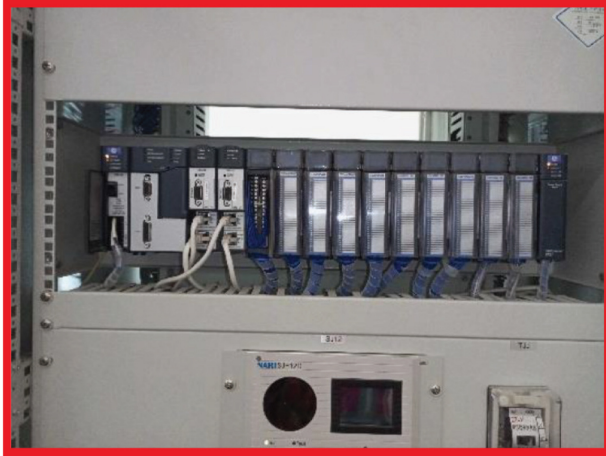
We Supply and Install PLC's
