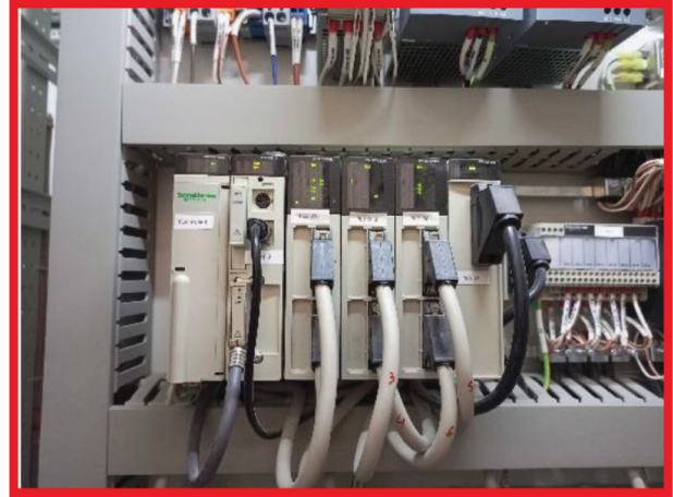
Brands from shneider, Mitsubishi, Siemens
